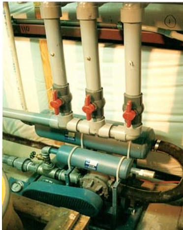
Compressor and Manifold for an Air Sparging System
