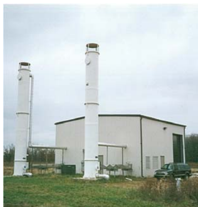
Air-stripping towers for groundwater treatment
